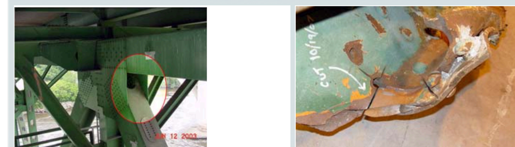
(a) Bending of a metal plate that was detected prior to the collapse. (b) Fracture that was later found to be a major cause of the collapse. Structural flaws of I-35W bridge
