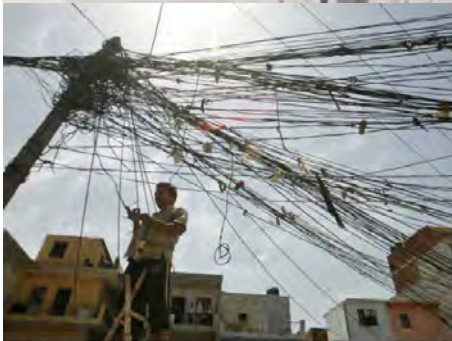
A man stands on a ladder to fix tangled overhead electric power cables at a residential area in Noida, India. April 4, 2013 (Reuters/Thomas H. Dreyer)
