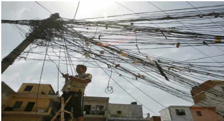
A man stands on a stepladder to fix tangled overhead electric power cables at a residential area in Noida, India, June 1, 2011 (Parivartan Sharma/Courtesy Reuters).
