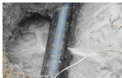
Water main breaks
