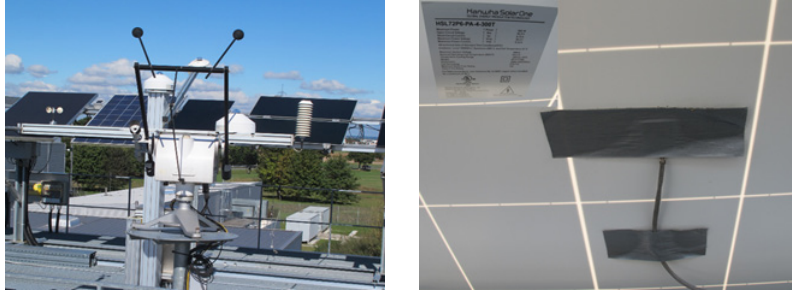
Figure 4: Weather station (on the left) and module temperature sensor (on the right).
