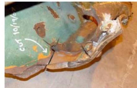
(b) Fracture that was later found to be a major cause of the collapse.
