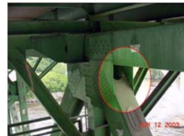
(a) Bending of a metal plate that was detected prior to the collapse.
