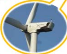
Wind Turbine Controls
