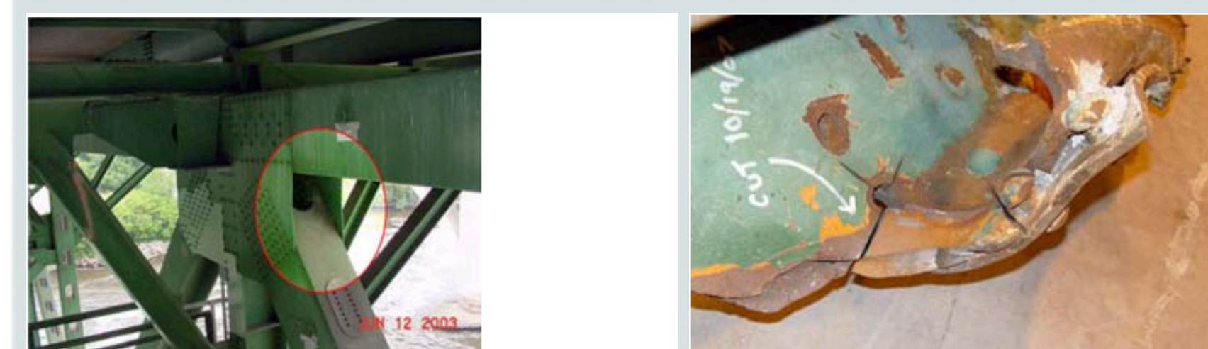
Structural flaws of I-35W bridge
