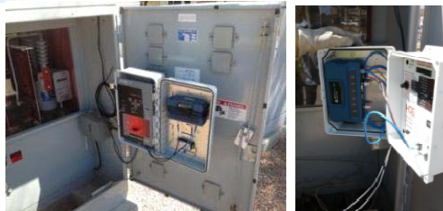
Multiple Communication Systems for Different Applications Two-way capacitor bank monitors and controllers, for Volt/VAR Monitoring & Control
