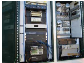
Data Acquisition System
