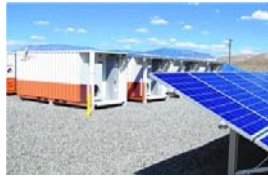
500kW PV and Advanced Carbon Battery for Shifting (1 MWh) and UltraBattery for Smoothing (500kW)
