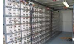
1 of 8 Containers Consisting of 160 Battery Cells Each
