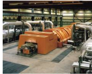
Power generation and distribution
