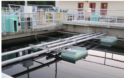
Maroochy Shire sewage plant (2000)
